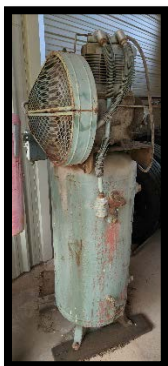
80 Gallon Air Compressor – Inoperable
