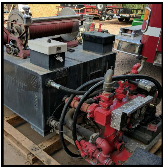
Skid Unit – 200 Gallon Tank/Hale Pump
